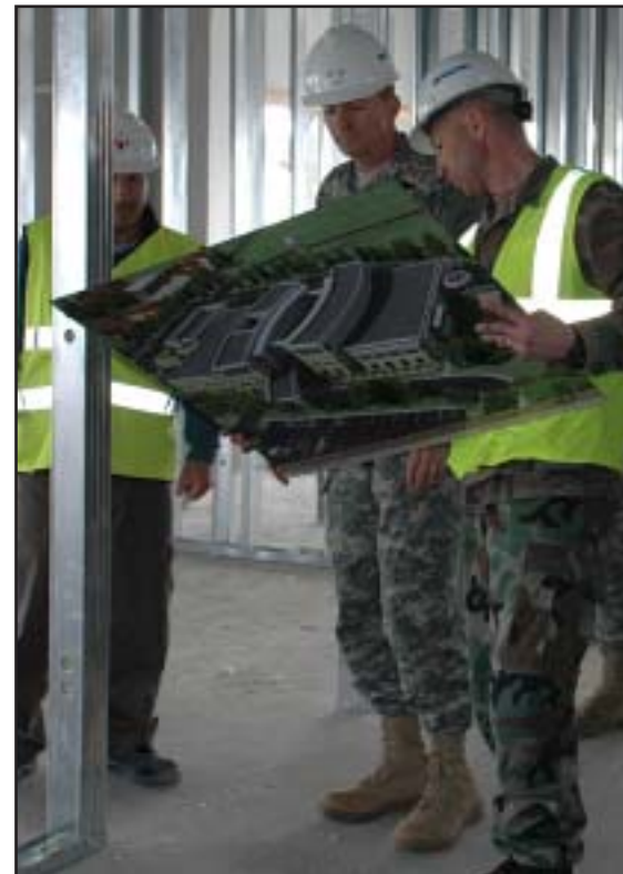
Cmdr. William Whitmire (right), U.S. Navy resident officer-in-charge of construction for the U.S. Naval Facilities Engineering Command (NAVFAC) Europe and Southwest Asia, shows Maj. Gen. William B. Garrett III, U.S. Army Africa commander, a blueprint of the layout of the new Enhanced Health Services Center during the general's visit to the construction site March 27. Assisting with the site visit was Frank Varano (left), project engineer with the Vicenza Health Facilities Planning Agency.
